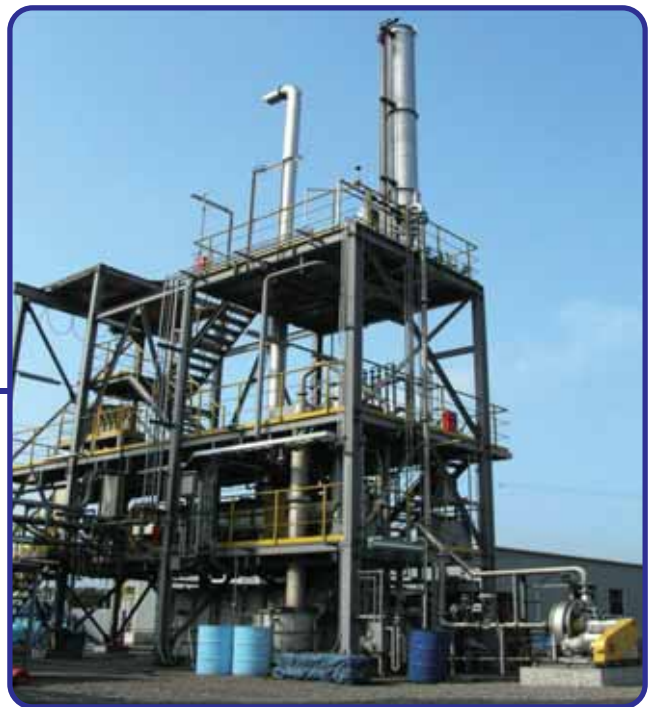
Process Development Unit for H 2 Production using Coke Oven Gas (The Japan Research and Development Center for Metals)
